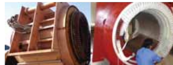
25,000HP, 13.8KV motor stator
